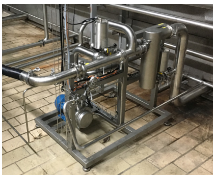
The eMotion unit is installed on a separate skid.
